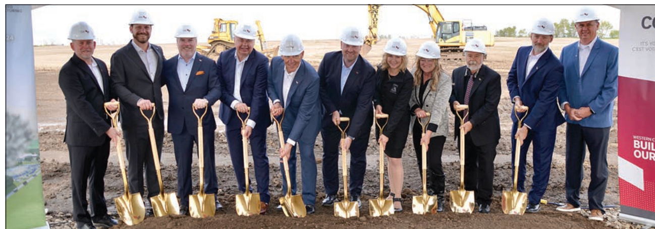
CGC broke ground for the construction of their wallboard manufacturing plant near Carseland on May 23.
