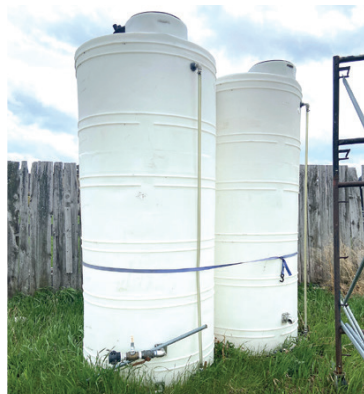
TWO 3,000L WATER TANKS Used for irrigation
