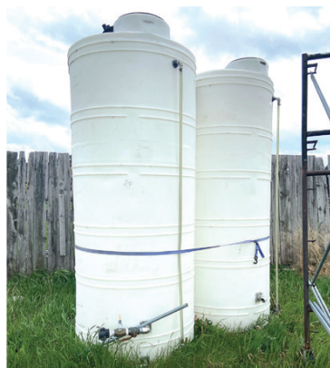
TWO 3,000L WATER TANKS Used for irrigation
