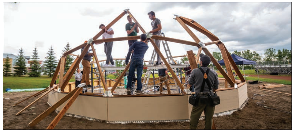
Teachers, students and community volunteers came together last week to construct the dome of the community greenhouse now presiding on SHS grounds. The frame of the structure, as pictured, was largely assembled on June 20.
