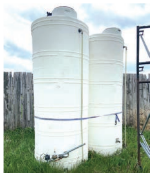
TWO 3,000L WATER TANKS Used for irrigation
