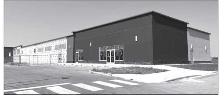
The new lab services building is currently being constructed in Edgefield. Mario Prusina Photo
